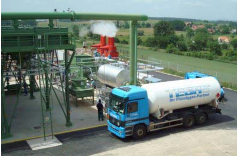
Figure 17: Soultz, France, 1.5-MW EGS Power Plant
