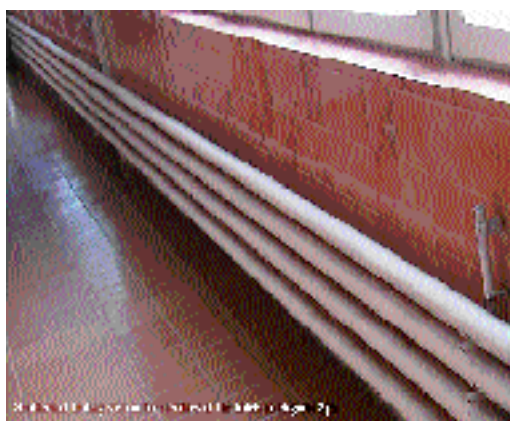
Fig.13. Characteristic parts of the Negorci Spa geothermal system: Heated complex of 5 spa buildings; Medical geothermal pool, and Characteristic heating installation for halls in the hotels part of the complex
