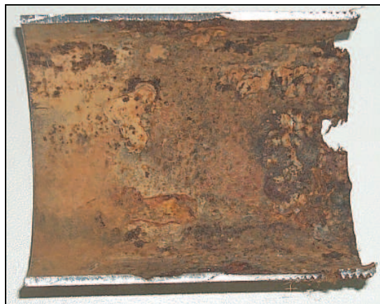
Figure 9.7. Picture of a corroded geothermal iron pipe section in contact a bronze valve.
