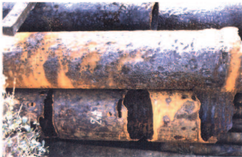
Figure 9.6. Underdeposit corrosion in carbon steel pipes from the villeneuve La Garenne
