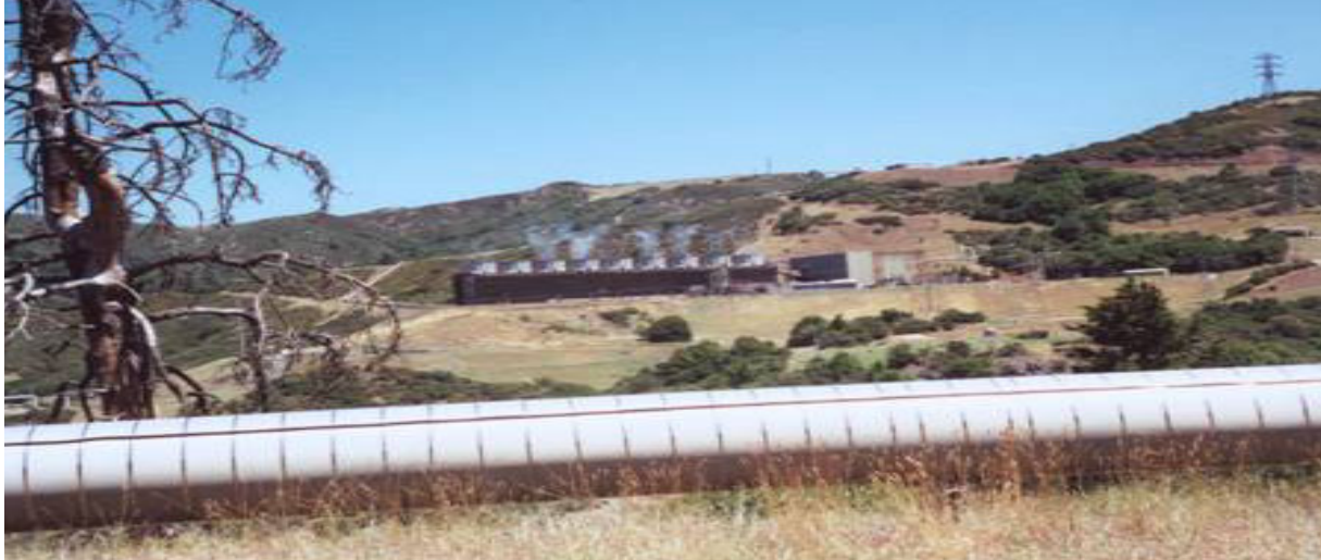
Figure 2. Eagle Rock Geothermal Plant one of 19 facilities operated by Calpine at The Geysers.
