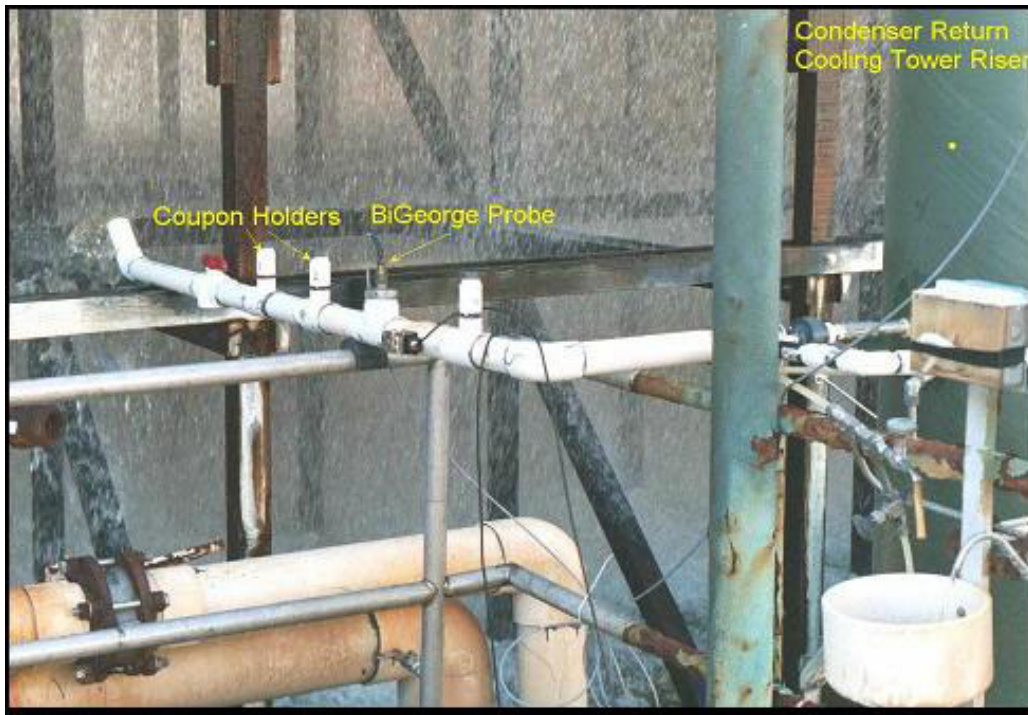
Figure 29. BIoGEORGE™ Biofilm Activity Monitor probe installed at the Aidlin Unit 1 cooling tower.
