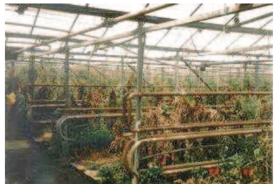
Fig.7.41. Aerial pipe heating system
