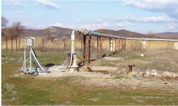
Fig.7.8. Aboveground geothermal pipeline in Smokvica, Macedonia (Popovski, 2000)
