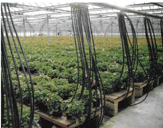
Fig.7.44. Bench heating with plastic pipes
