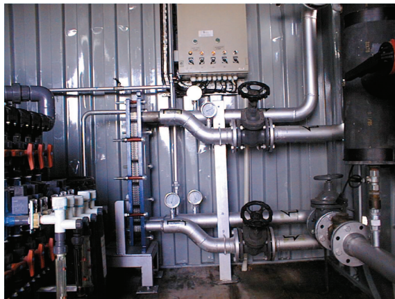
Fig.7.16. Connection station of the greenhouse complex in Ribeira Grande (Azores, Portugal)
