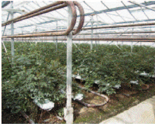
Fig.7.42. Combination of aerial and vegetative heating installation for growing roses
