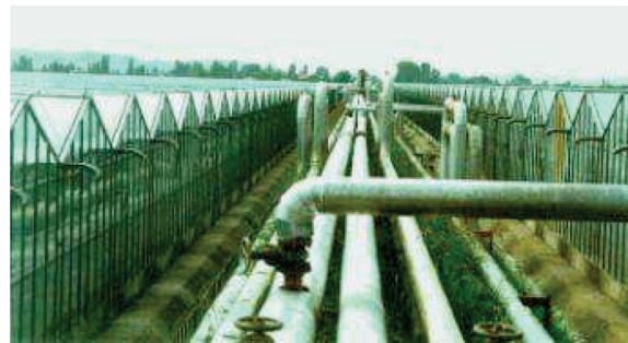
Fig.7.10. Properly completed distribution pipelines for large complex of geothermally heated greenhouses (Kocani, Macedonia)
