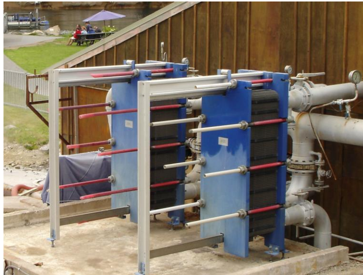
Figure 3.2. Plate heat exchanger at the Taupo Prawn farm (Thain et al 2006)
