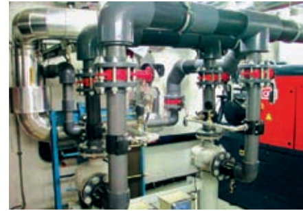
Heat pump for industrial use in DePuy factory, Lyon, France
