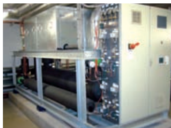
Large ground source heat pump (ca. 400 kW) and manifold for larger project
