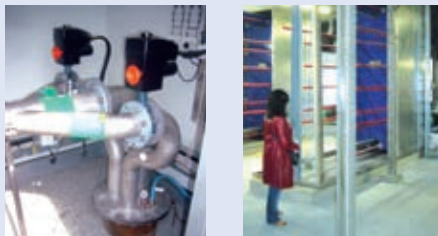
One well and the heat exchangers of the ATES for Arlanda airport, Sweden
