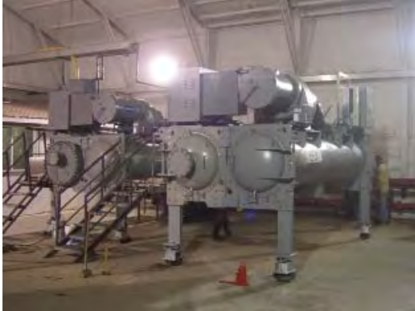
Figure 22. ORC #1 (background) and ORC #2 installed in the power plant building
