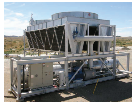
Fig.7.3.2 Ormat ORC binary cycle power plant
