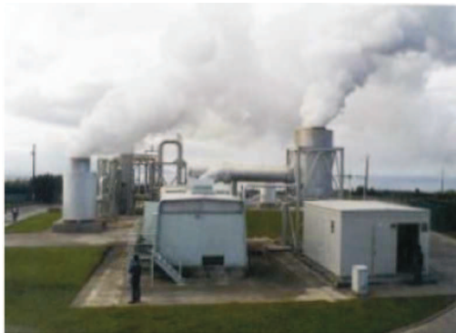
Fig.7.1.1 Direct-intake, non-condensing single flash geothermal power plant at Pico Vermelho (São Miguel Island, Azores) exhausting steam to the atmosphere. (source: 2004 Lund).
