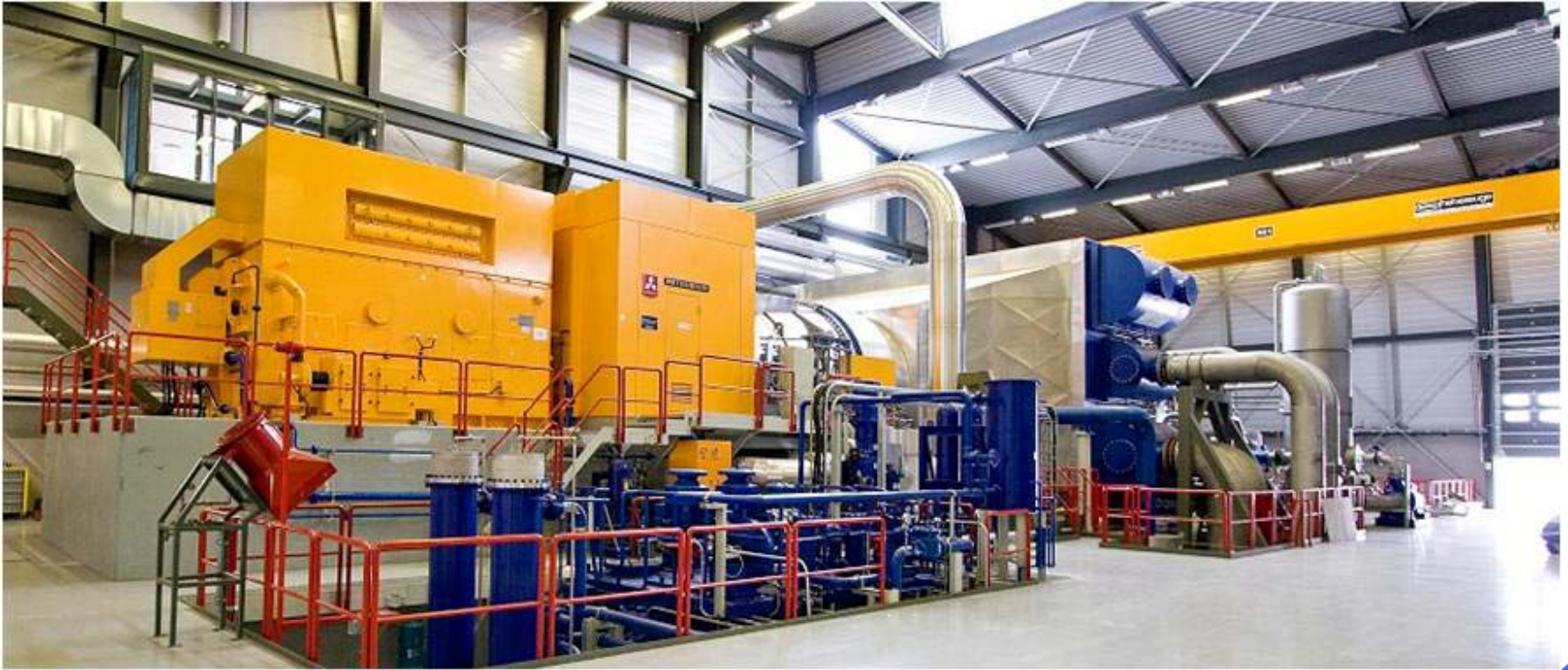
Hellisheiði power plant
