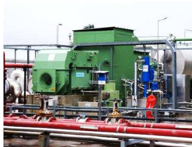
11 kV Asynchronous generator (12.000 rpm) and gear box
