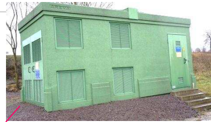
20/0,4 kV transformer station
