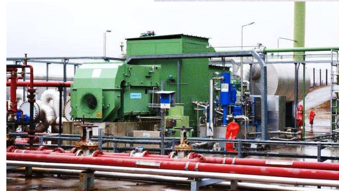
generator (12.000 rpm) and gear box
