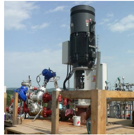
view at well head/motor
