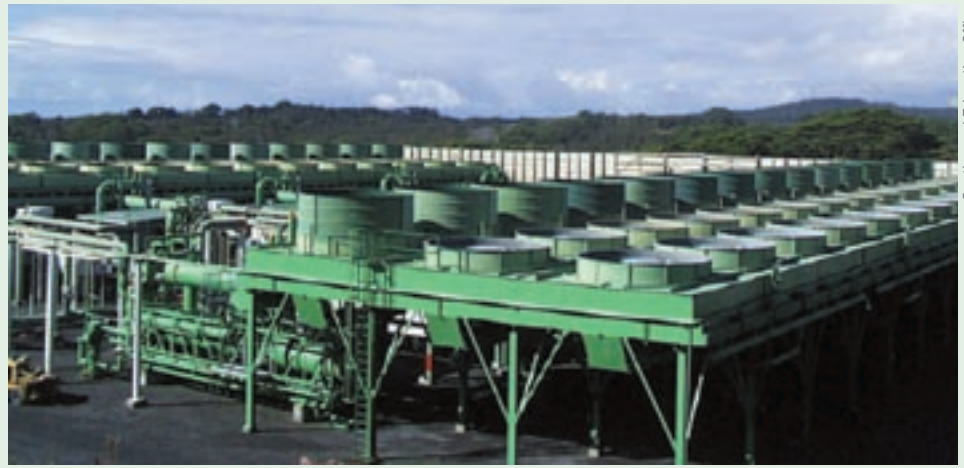
This 30-MW, air-cooled geothermal power plant on the Big Island of Hawaii (Puna) blends in well with the natural landscape.
