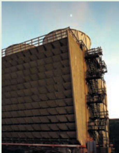
Geothermal power plants use cooling towers, like these at The Geysers, to safely reject waste heat into the atmosphere.
