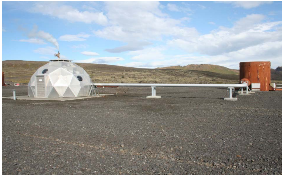
Enclosed wellhead connected to a muffler
