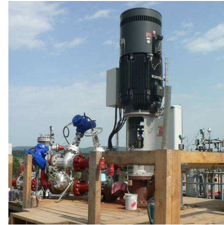
view at well head/motor
